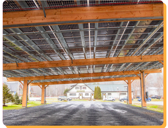
Solar Canopy, Lawson's Finest Liquids, Vermont
